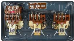
Interior View of MK2 SASD
